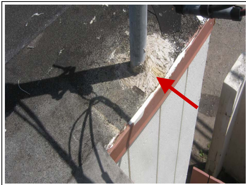
1907-003B-A19: White Caulking on Pipe Penetration with Black Mastic Building B Studio Roof
