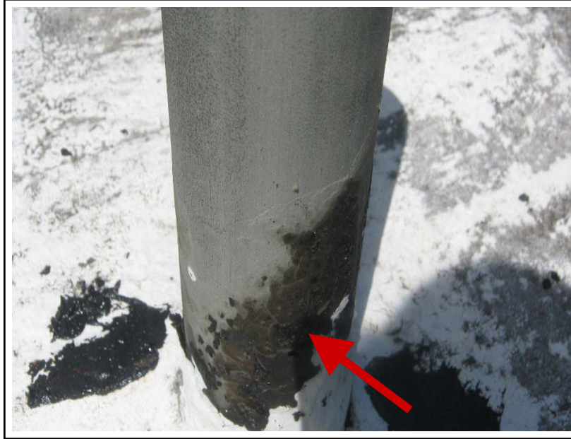
1907-003B-A04: Black Mastic on Pipe Penetration Building B Studio Roof
